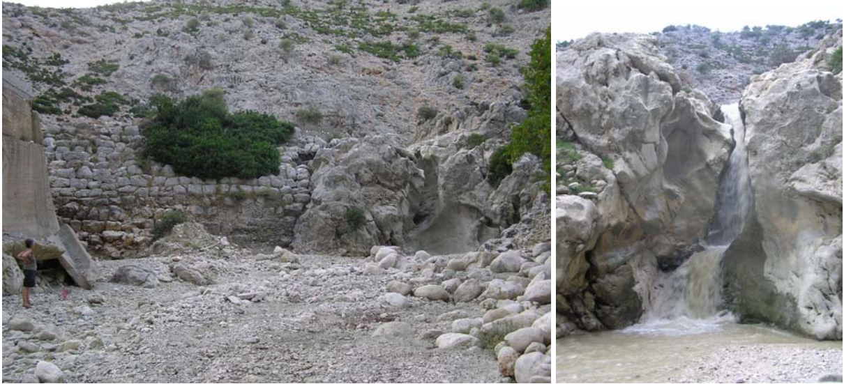
Figure 7 The dam of Alyzia; the spillway with its irregular shape formed by erosion through centuries is shown on the right of left photo and in operation in the right photo.
